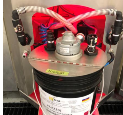
Safety key out (Section will flash)
